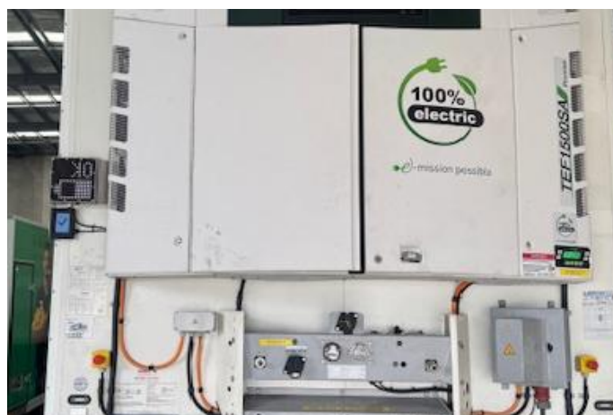
Figure 7. Example of Battery Status Indicator digital display
